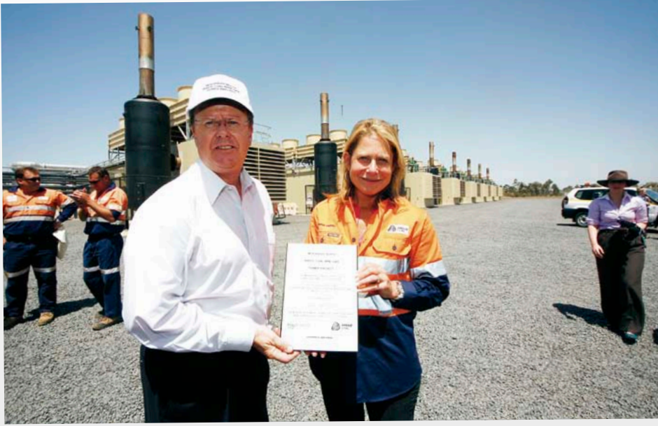
Minister for Mines and Energy Stephen Robertson MP and AAPlc Chief Executive Cynthia Carroll present the plaque at the Moranbah North WCMG power station.
