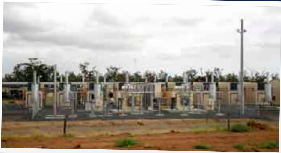
ACA's 32 mega watt power station uses coal seam methane from Capcoal.
